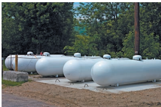
Photo 7.3 Cylindrical pressure vessels.
